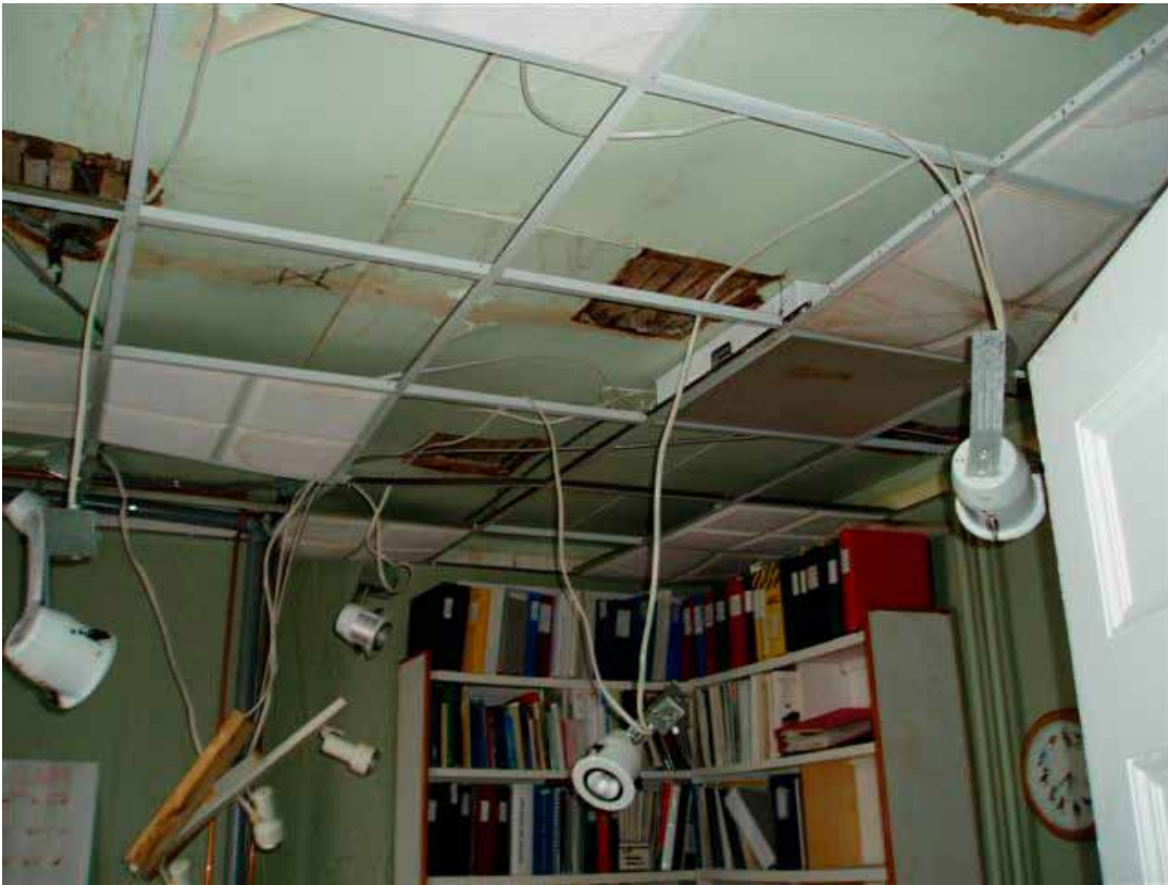
Water damage to the Coalition office following the burst pipe in December 2009. Photo by James Tweedie.
